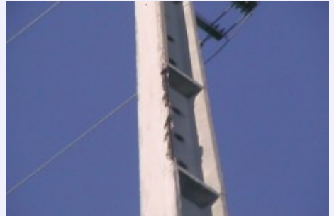
Visual detection and classification of equipment defects
